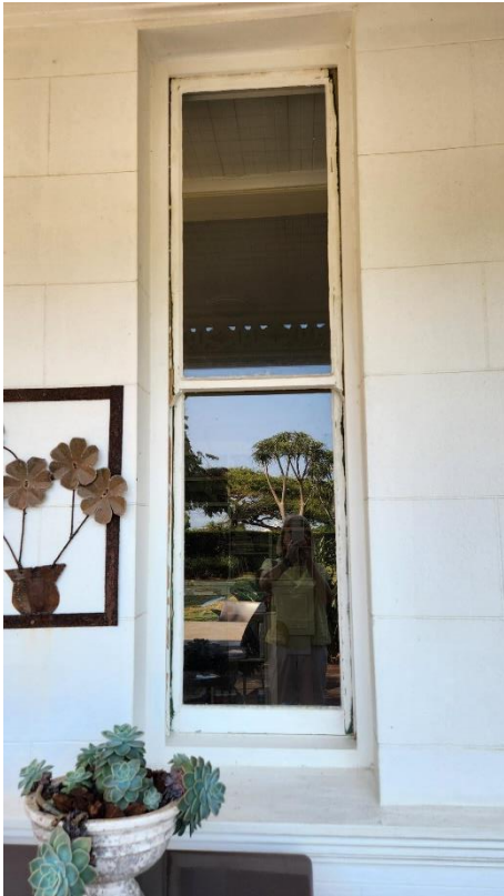
The original sliding sash windows require continuous repairs and maintenance.
