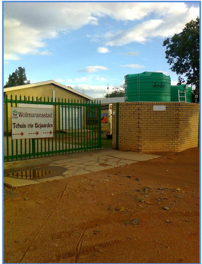
Plate 5: View of water storage infrastructure erected at the Wolmaransstad Old Age Home as part of borehole infrastructure
