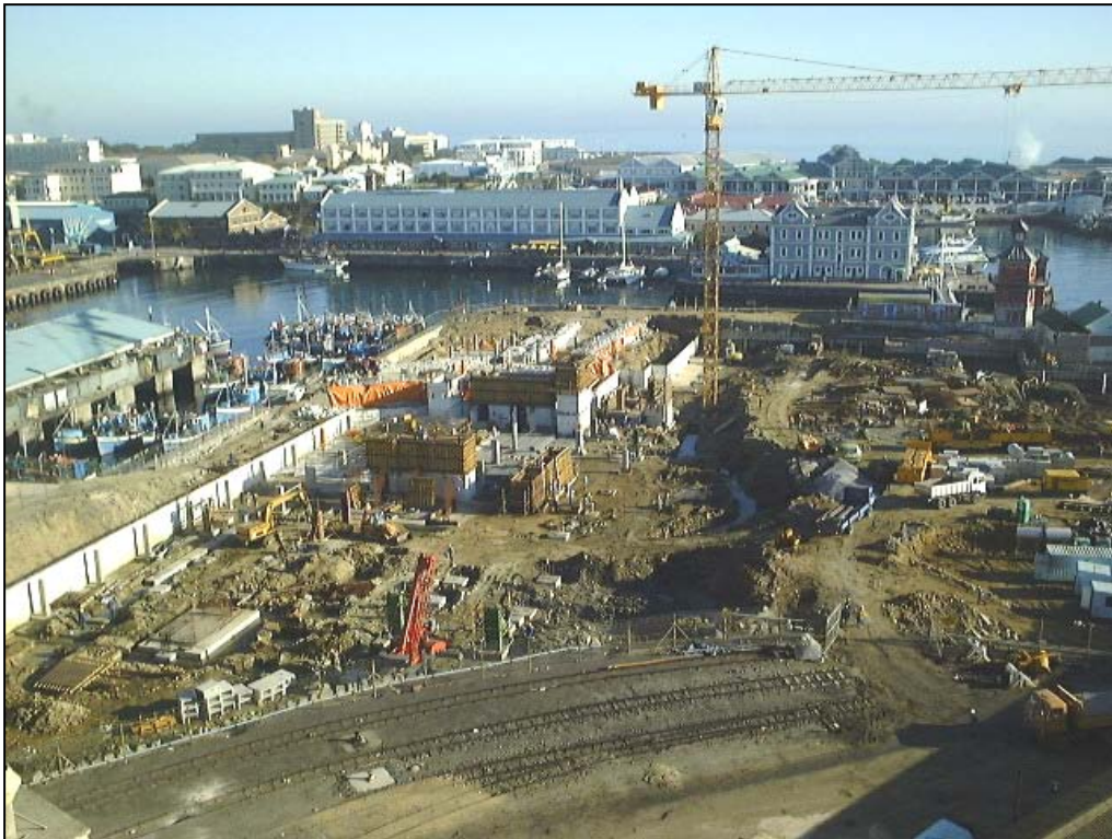
Figure 9 The site of the Chavonnes Battery (left of crane) is encased by a retaining wall and protected by orange plastic covers and sand bags. Excavation of the underground parking level is in progress.
