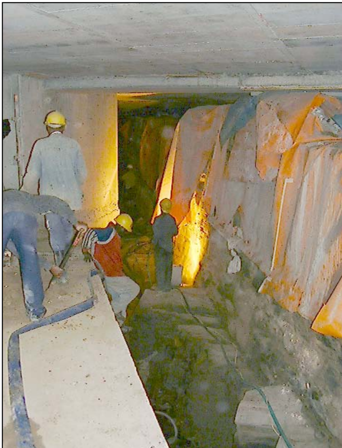
Figure 11 Workers prepare to remove the protective plastic covering before cleaning the south wall and rocky seabed.
