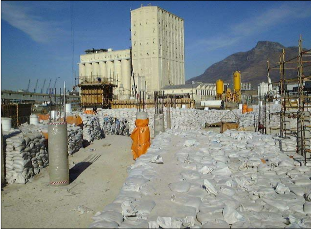
Figure 10 Original fabric has been protected with sand bags prior to construction of the BOE building. Columns are being cast well clear of the Battery walls.
