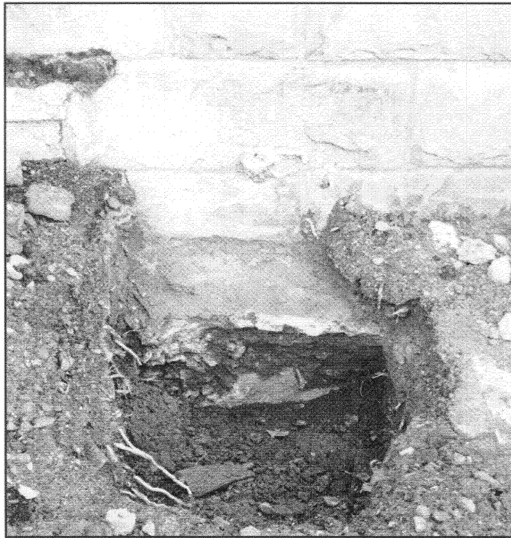
Plate 16: The concrete foundation at the foot of the wall of the Varsity College Building.
