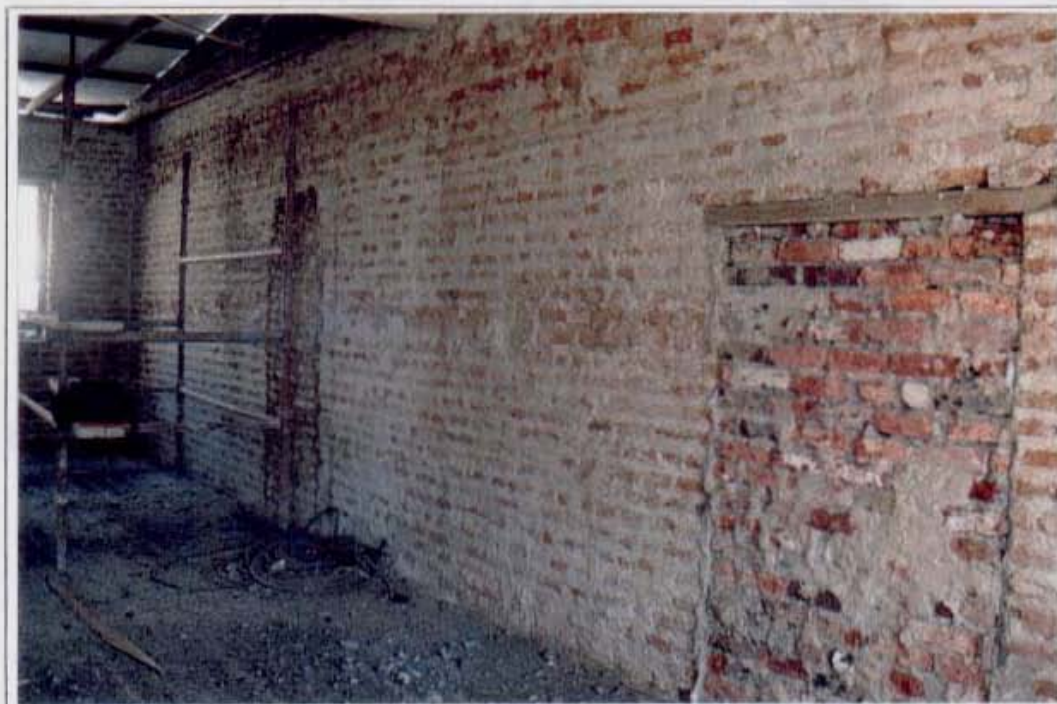
PLATE 7: All of the brickwork on the second floor post-dates the turn of the century although extensive use has been made of recycled 18th and 19th century fabric.
