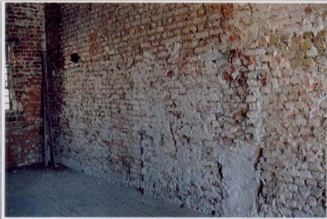
PLATE 6: First floor: the remains of the internal dividing wall is visible as a scar (right), while the change in brick work texture indicating a height raising event (1902) is indicated by an arrow.
