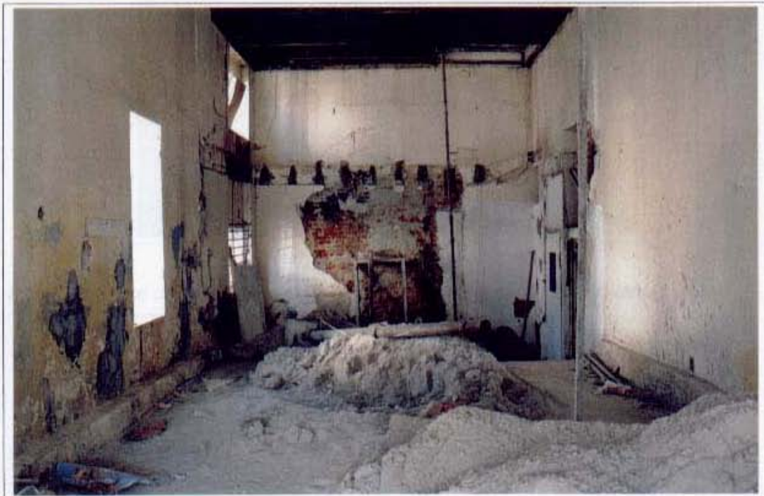
PLATE 2: Interior view (Hout Street side) showing soot blackened 18th century fabric, and beam slots (possible opkamer above).
