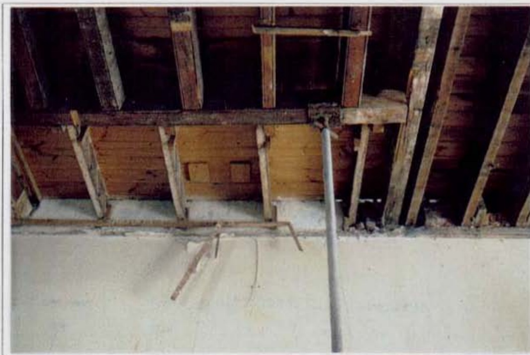
PLATE 4: 18th Century beams (Hout Street side) reused along with 19th-early 20th century pine.
