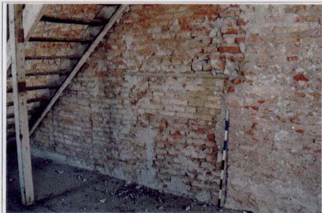
PLATE 5: Interior view, (Hout Street side) first floor showing early openings projecting through present (1902) floor levels.
