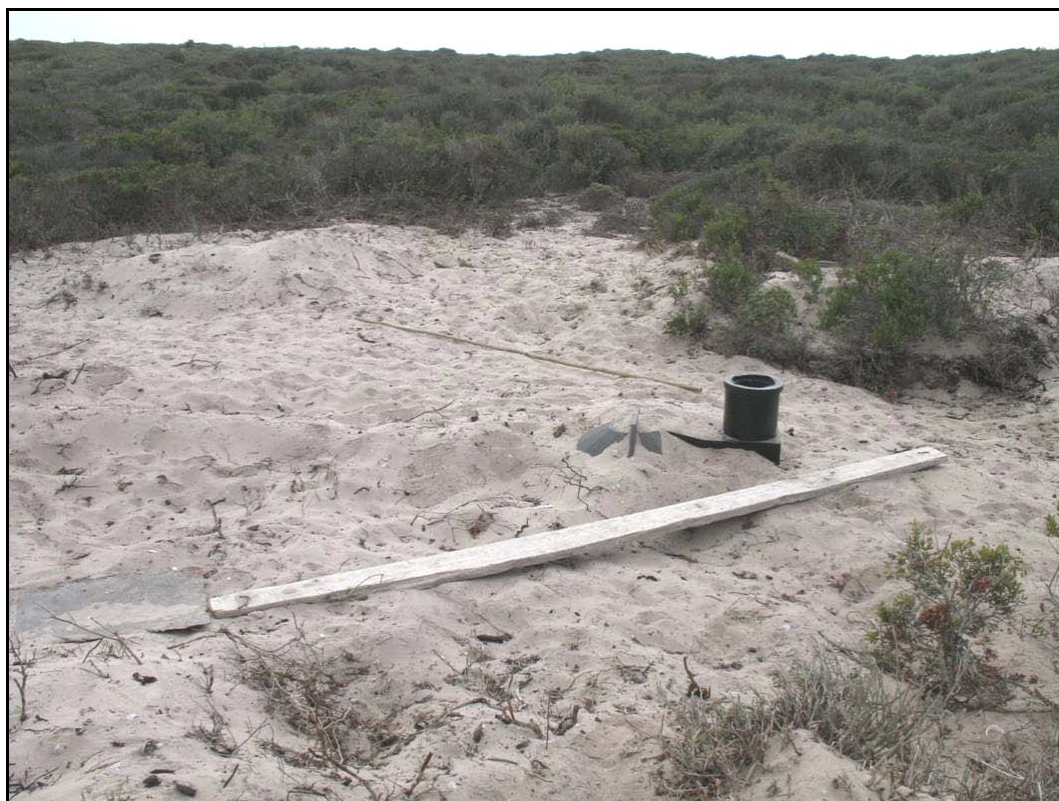
Figure 7 : The septic tank in place at Point F. Note the lack of shell in the churned up sand.
