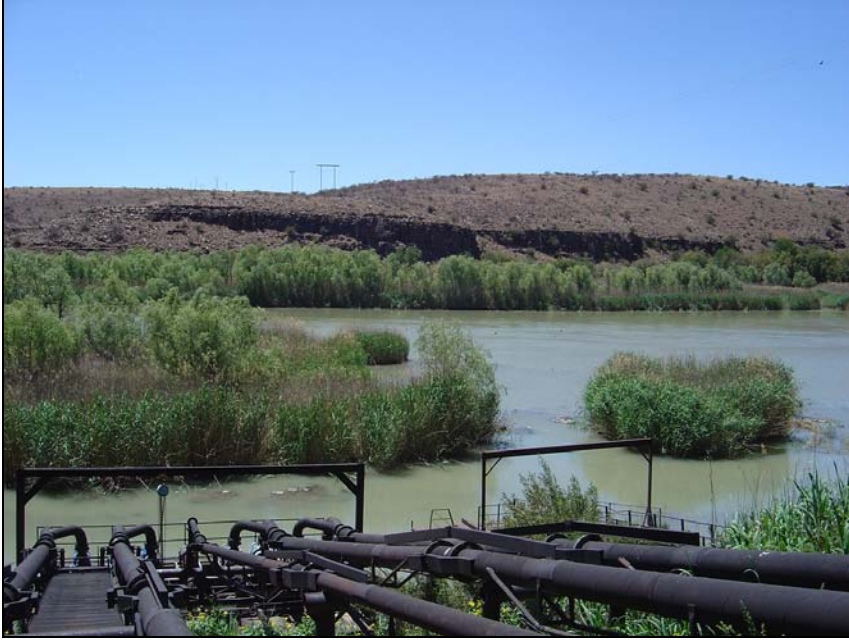
Fig.13 (6) The locality on Zuurgat 82 where the power line will cross the Orange River from Wiclow 218 on the opposite side. Existing pump installation in the foreground.
