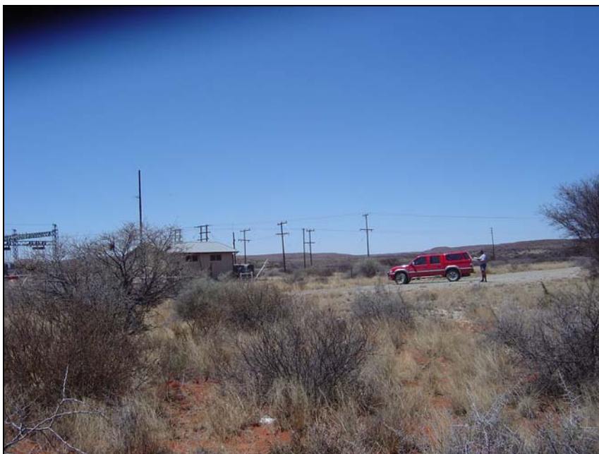
Fig.15 (8) Disselfontein Substation where the proposed new line will join the existing ESKOM power line network.
