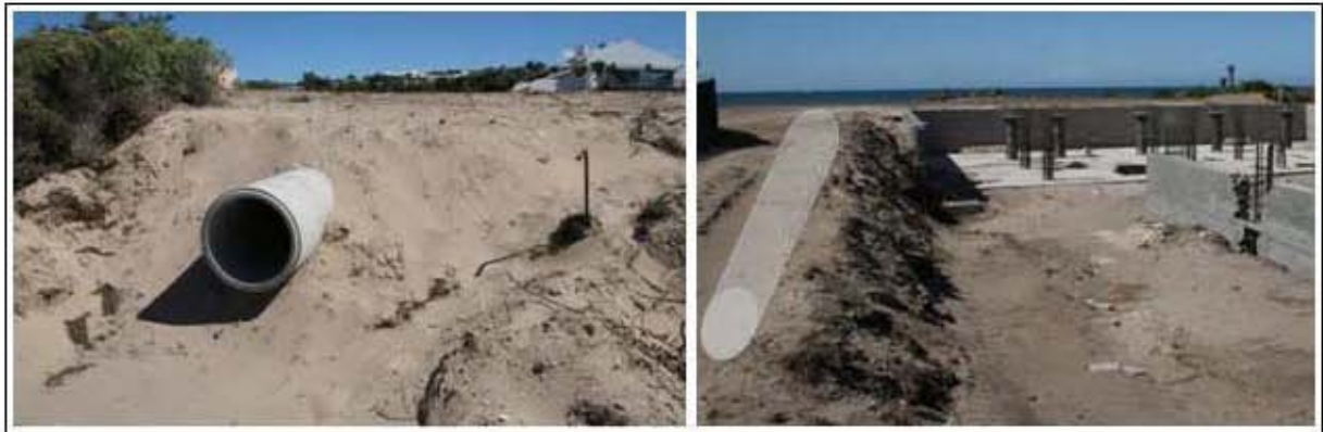
Plate 6. Location and trajectory of storm water pipeline along northern extent of property. Left image taken from east (beach) and right image taken from west (road) with schematic placement of pipe in grey.
