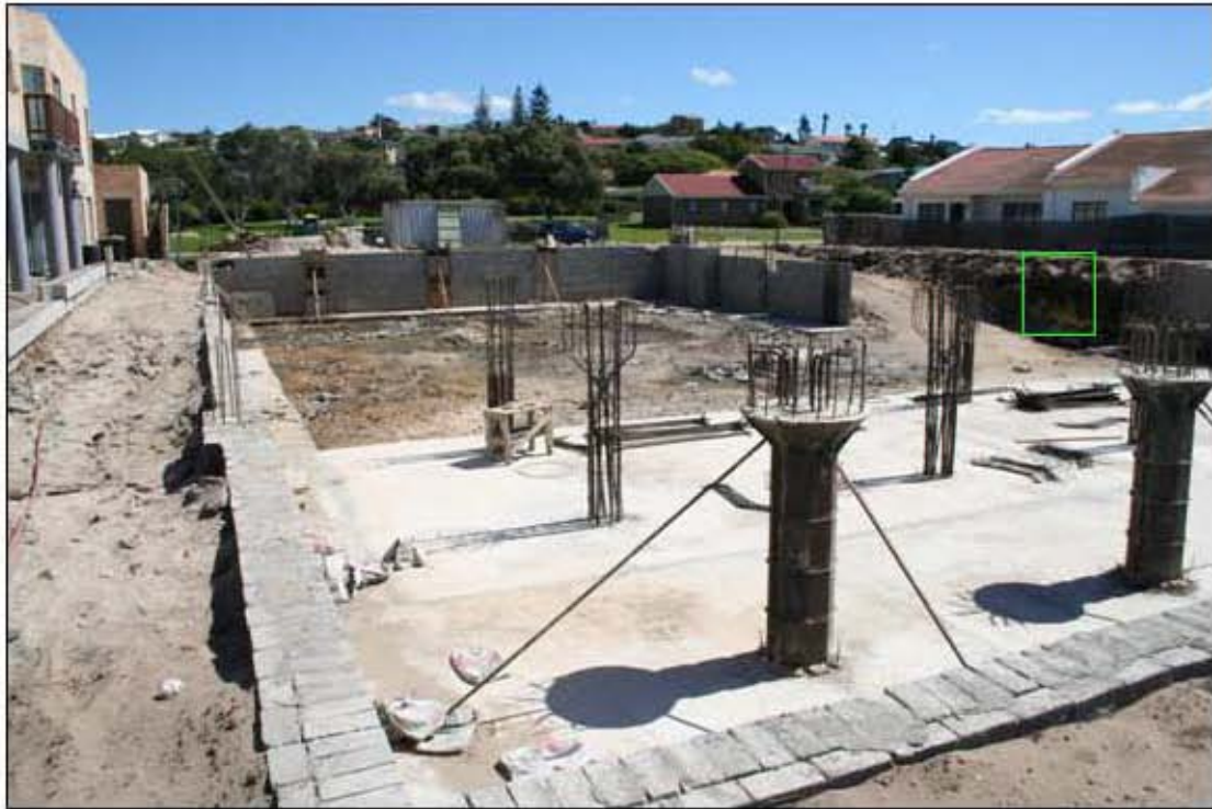
Plate 3. Basement and footprint of new structure in western portion of property (see Plate 2). The profile shown in Plate 4 is framed in green.
