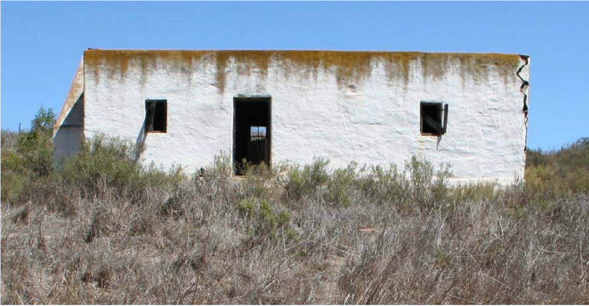
Figure 3. Worker's cottage on the property - note the crack in the end wall.
