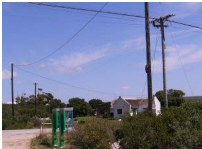
Fig. 4. Wooden poles carry power to ‘Huis 31’ and other cottages. The main Eskom line along the R305 in the foreground is also on wooden standards.
