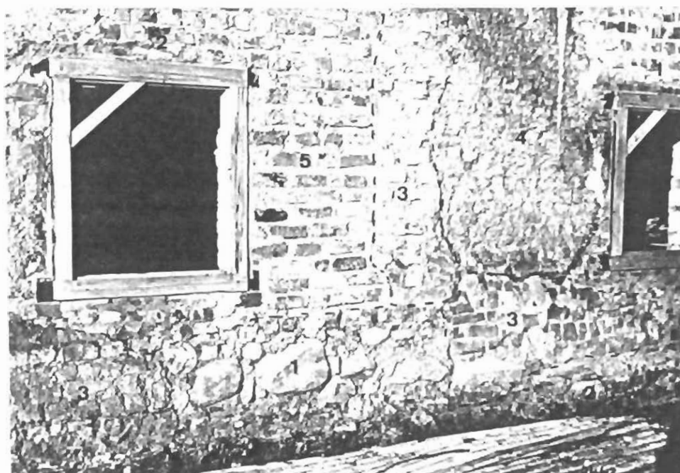
5. Close-up of the right portion of the façade wall between window 1 and window 2 (Rooms CC/C). Note the old foundation of river stones (c.1800?)(1), granite (c.1740)(2), brickwork (19 th century)(3), the c.1740 raw brick (4) and 1975 fill-in brickwork and windows (5) (Le Roux 1974)
