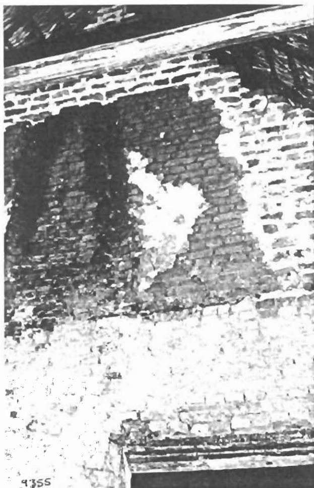
35. Wall D2 showing the difference in clays and raw brick colour of the lower and upper portions, indicating different periods of construction. The old lintels are still in position (Le Roux 1975).
