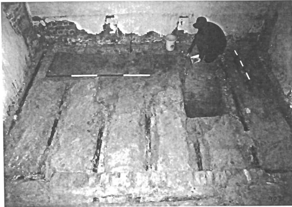
58.3 View of unit C with its joists. Note the extra joist behind the excavator, parallel to the 1m scale. It serves as proof that there was once a doorway here. The 2m scale is in line with the old >1760 hearth wall. The test pit (section C) was dug in 1981 (looking E).
