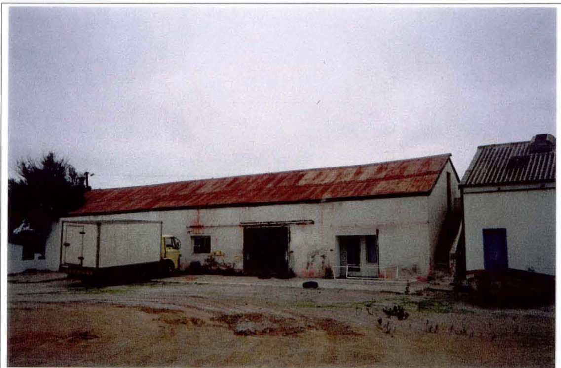
PLATE 2: Shed (A on Figure 2). Built with dressed limestone and with structural features which suggest that originally the roof would have been thatched.
