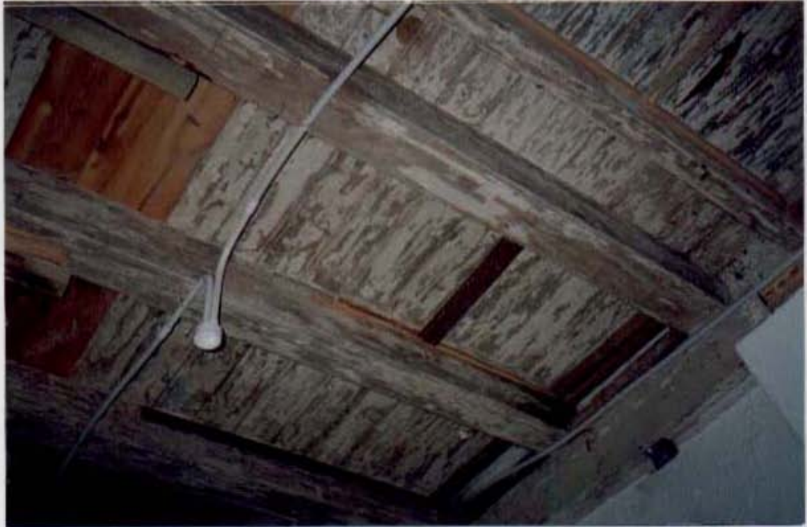
Plate 1: Photograph illustrating some of the yellow-wood beams in the ceiling dating to between the late eighteenth and early nineteenth centuries.
