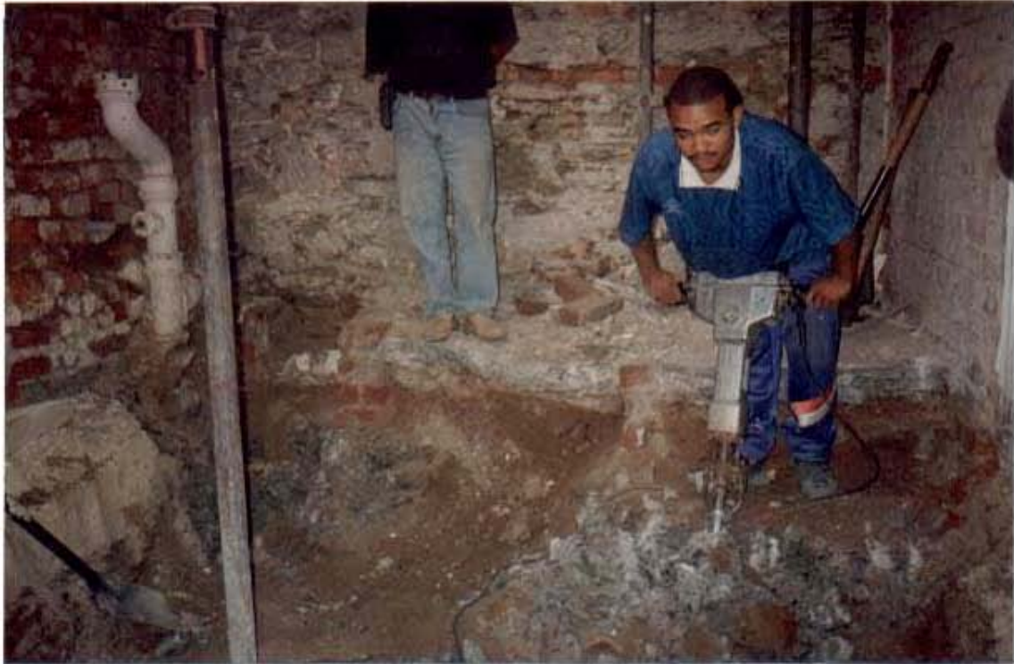
Plate 3: Photograph illustrating the disturbed nature of the deposit. The contractors in the photograph are breaking up the foundations for the toilets built in the courtyard.
