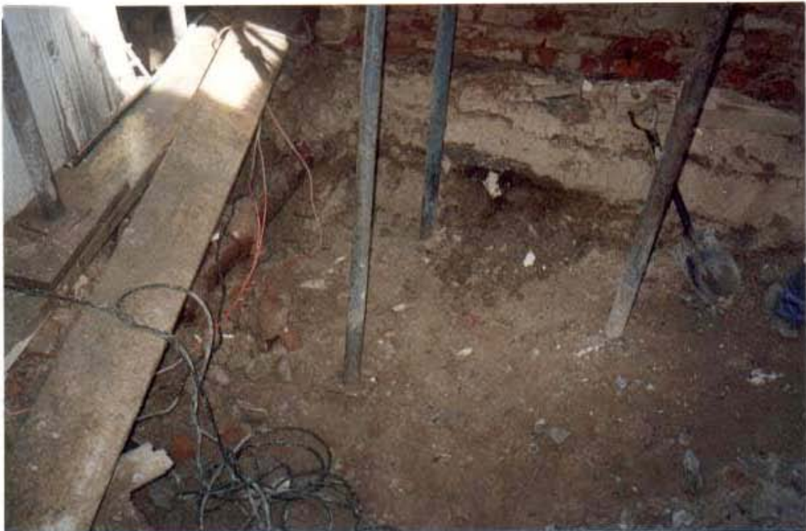
Plate 4: The position of the test excavation (parallel to the planks in the photograph). Note the pipes intruding deep below the surface.
