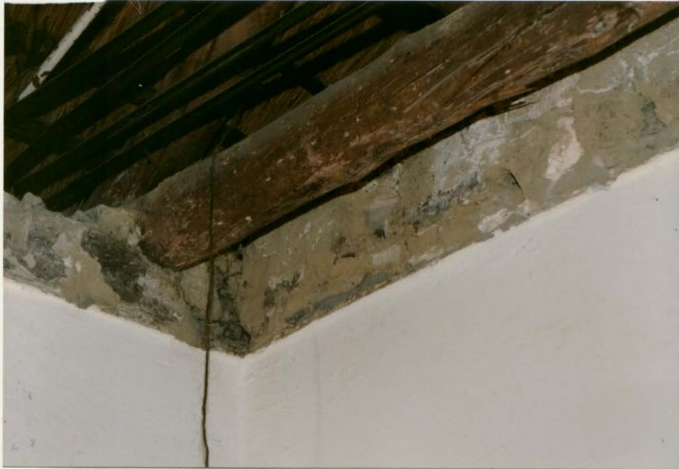
Figure 3.11: Beam and older plaster.
