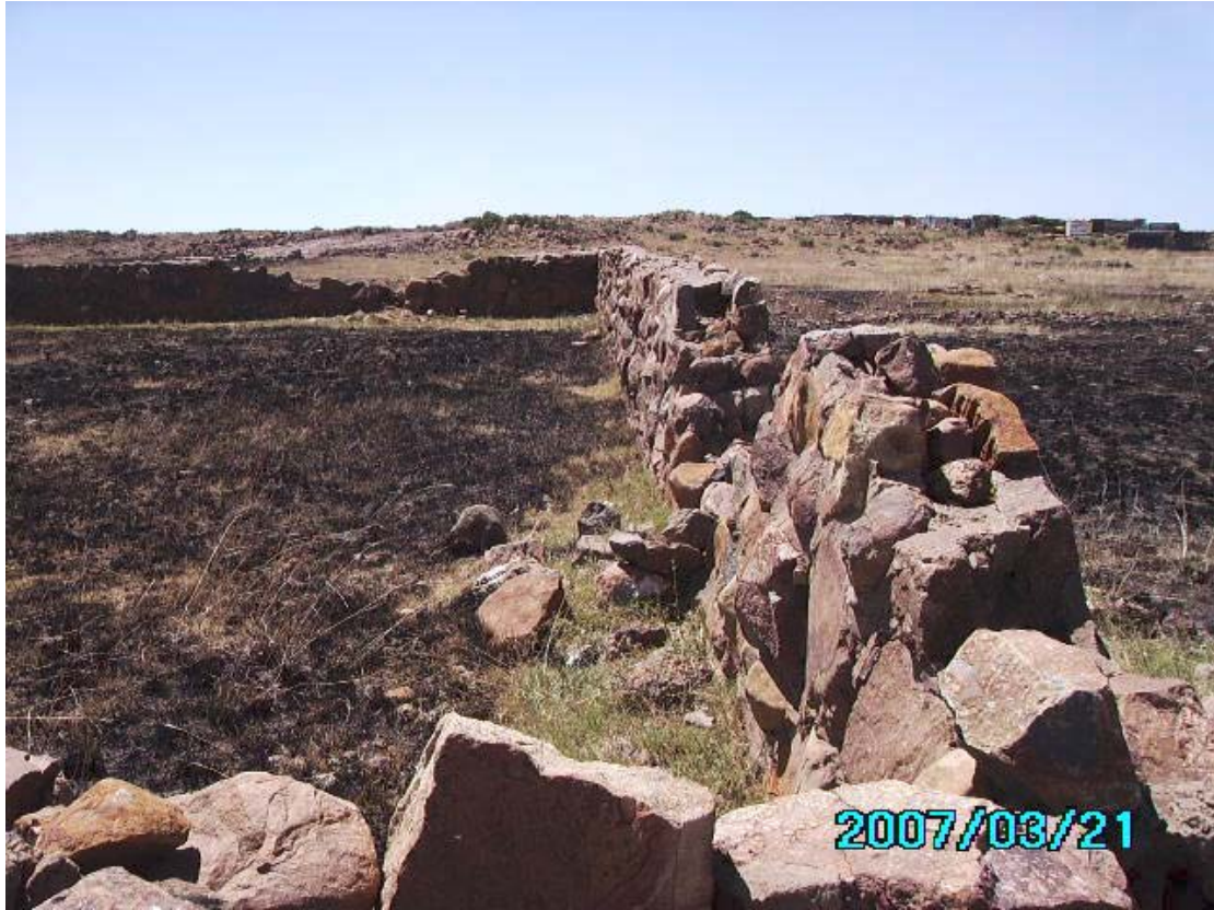
Figure 10. The wall of the kraal is built of stone but cement mortar was used as binding material.. There is no apparent reason why this should be preserved.
