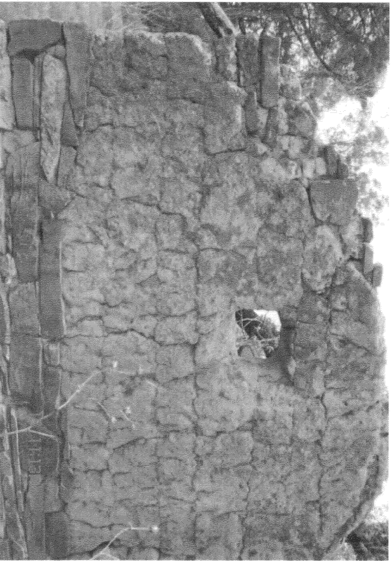
No 2 Detail of gable of 1860 house with layers of clay clearly visible
