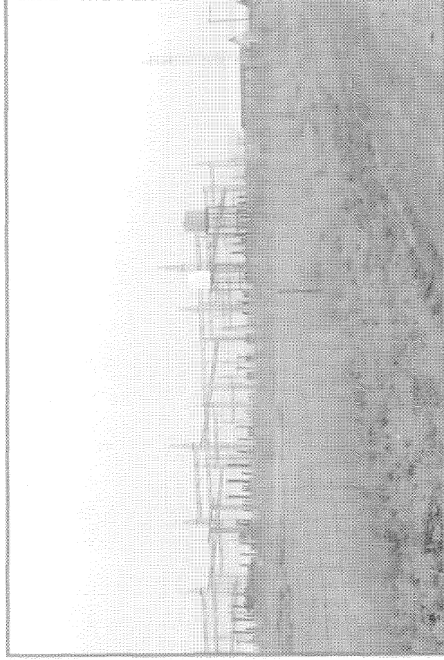
Plate 1: Proposed powerline will begin at this Machadodorp Eskom Substation 132/22/11KV
