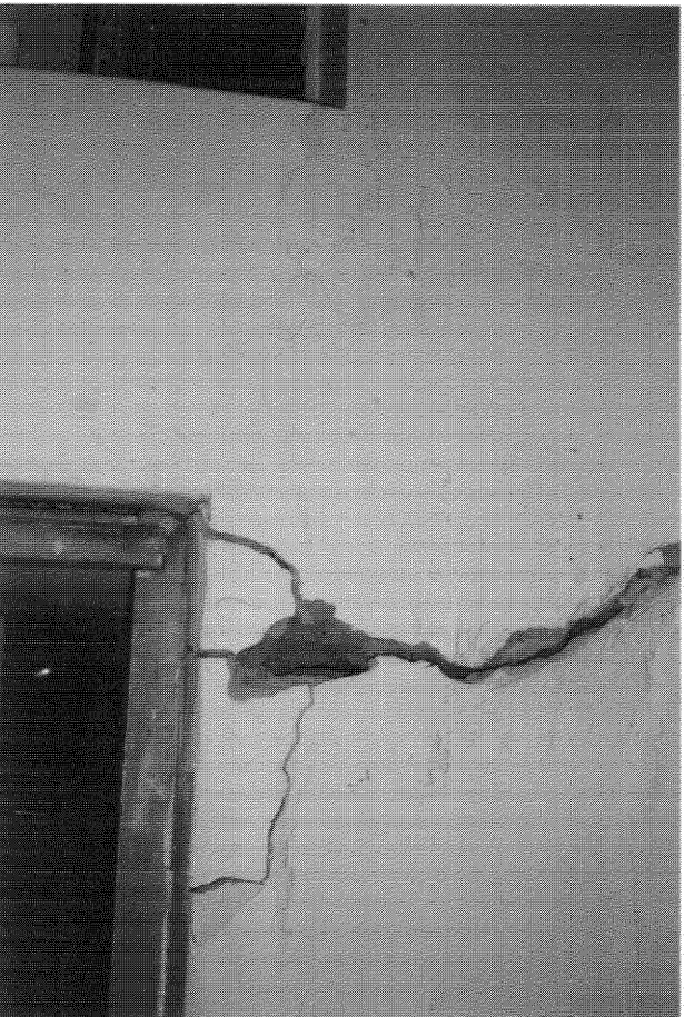
Fig 6. View of the cracks which are threatening the house.
