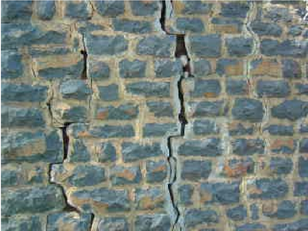
No 8. Cracks in the northern wall of the house
