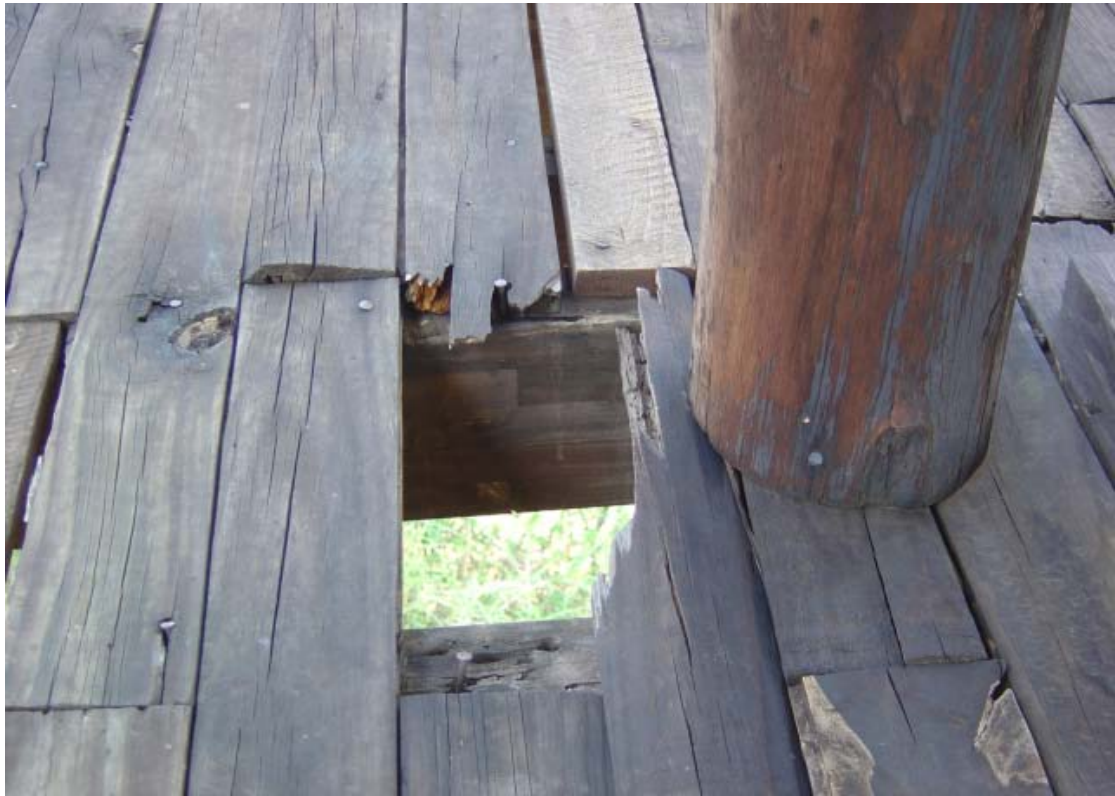
No. 5 Rotten floorboards of the viewing platform
