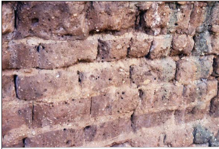
Fig.13 The wall of a little mining house dating from the 1800s, built of raw clay blocks.
