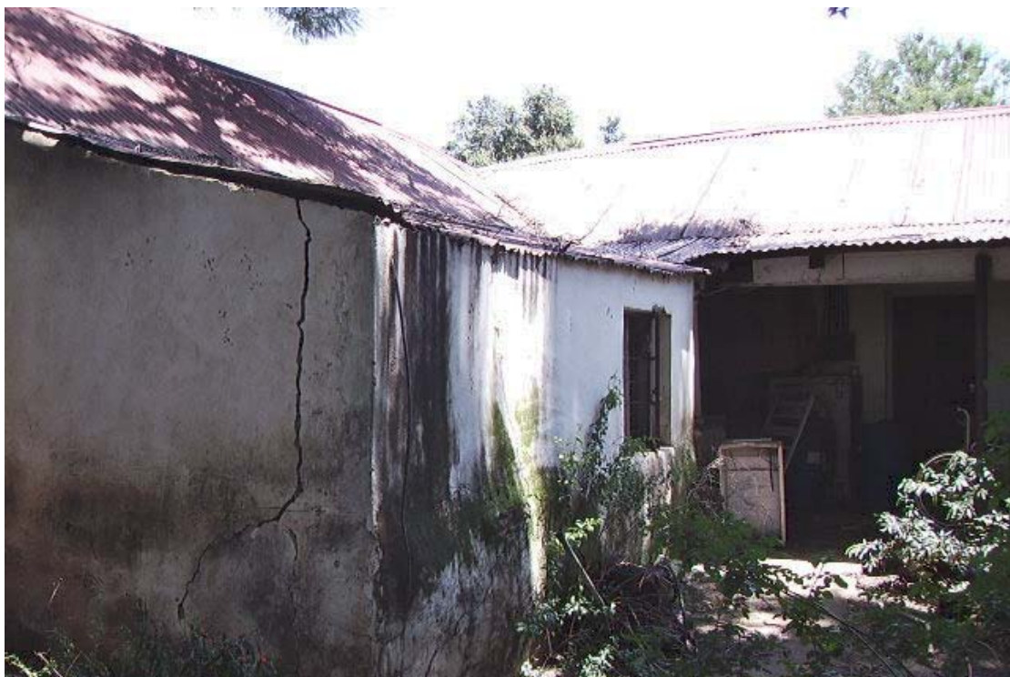
Figure 13. The eastern wing of the 1910's house. This veranda was also enclosed at a later stage. The workmanship was of poor quality.
