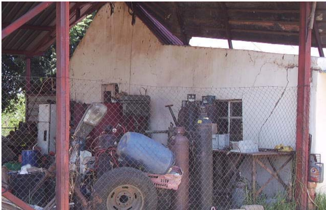
Figure 09 The northern side of the 1910's house with the effect of the workshop and machinery that does not help for the preservation of the building.
