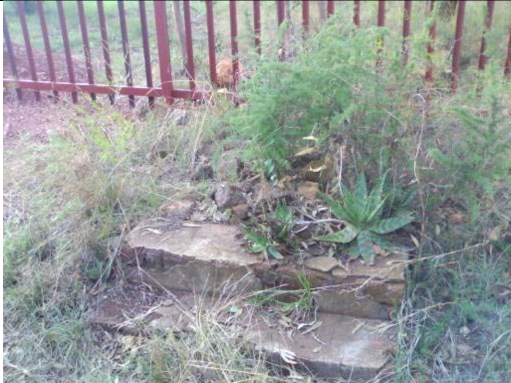
Figure 6: Damage caused by fence
