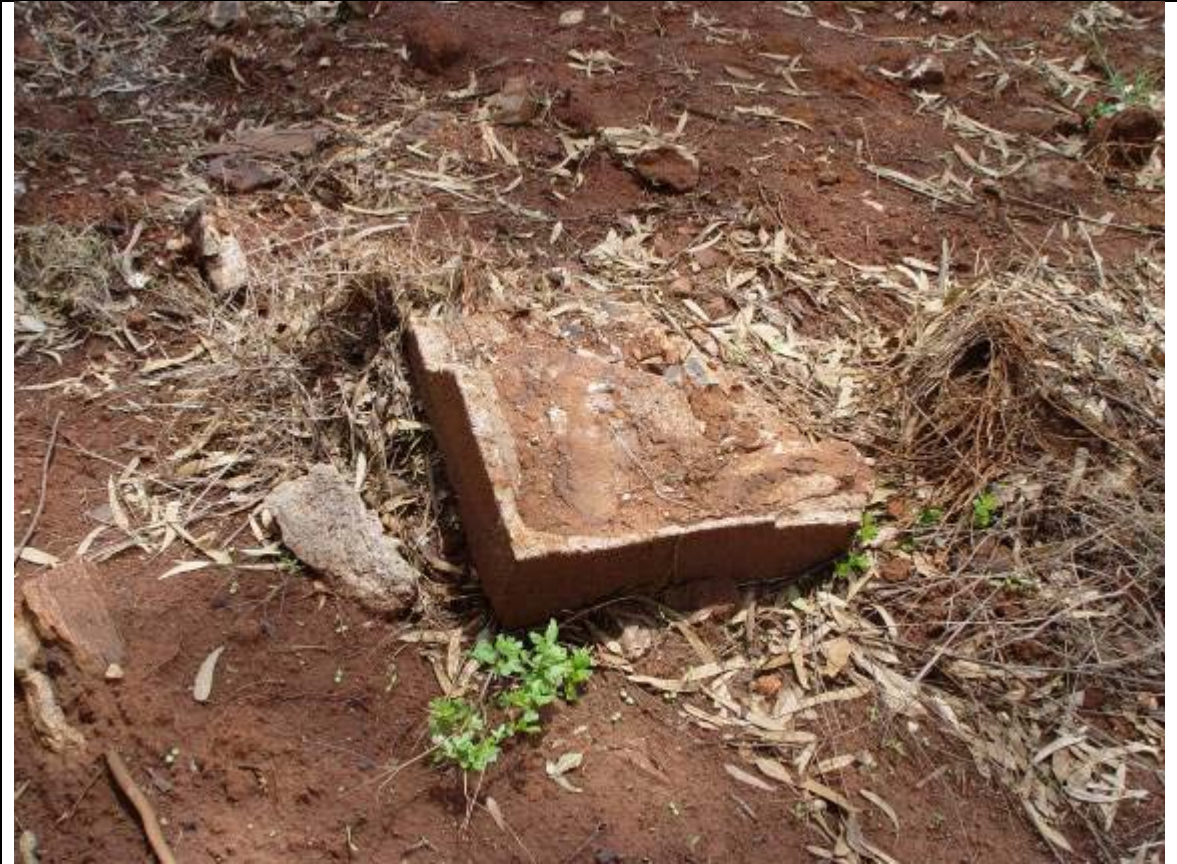
Figure 2: Damaged caused by the trench to Structure O
