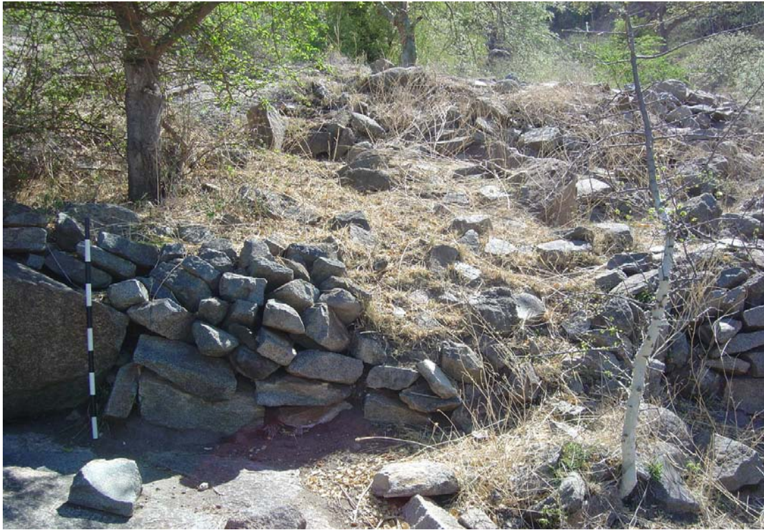
1. Partially collapsed walls on Mosego
