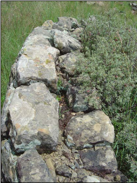
Fig.7 The walls are still in a very good and sturdy condition. The building method seems to indicate construction by a European-builder.
