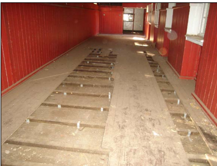
Fig.8 The extent of the vandalism is becoming serious.
