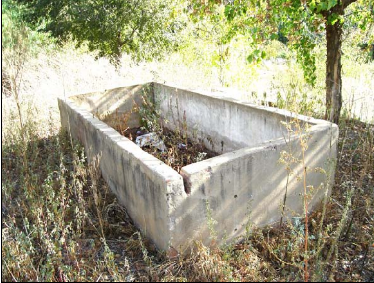
Fig.53 This concrete feature known as a “mist-propagation bed”, part of the PWD nursery.
