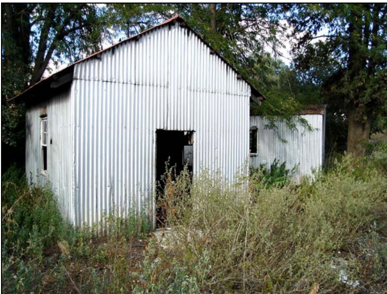
Fig.42 Small corrugated iron structure used as rest room by labourers at the nursery.
