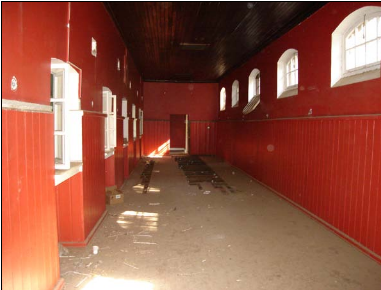
Fig.7 Interior of the Stables. Floorboards are vandalised by roaming homeless persons.
