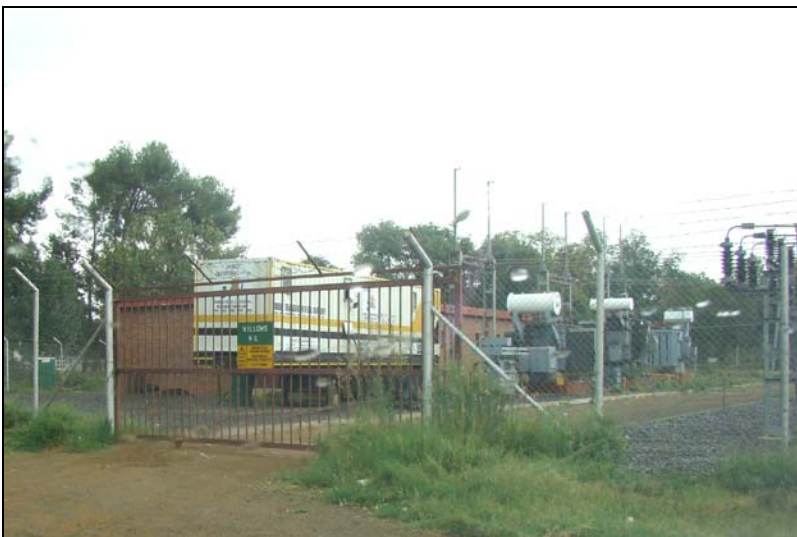
Fig.7 Point E Sub-station at the corner of Park Road and Parfit Avenue.
