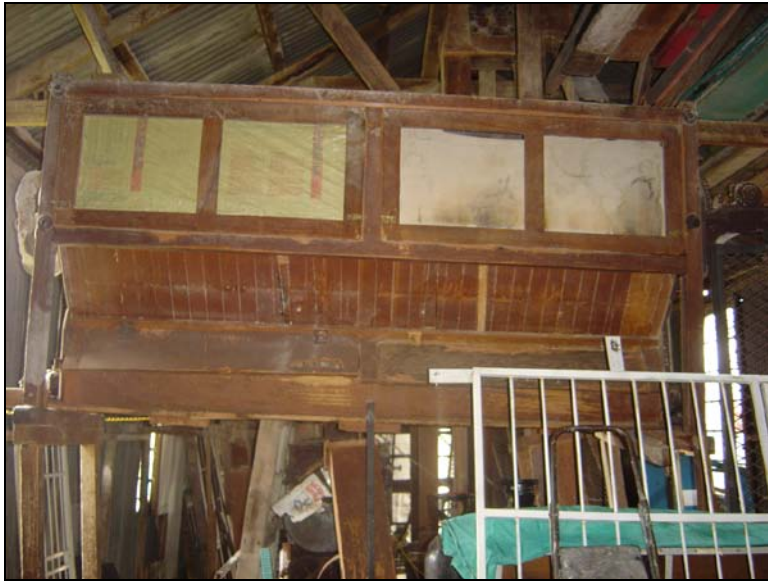
Fig.9 Some of the milling equipment which are still in place.
