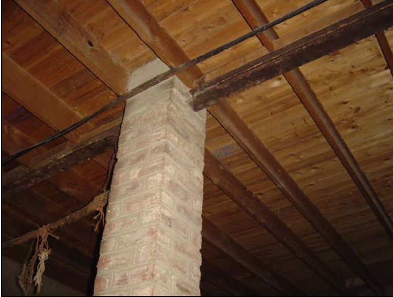
Fig.5 A brick column which carries the beams and wooden floor of the first storey.
