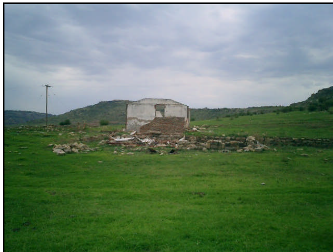
Figure 16: The complex of 4 outbuildings, in varying stages of decay, related temporally to both the origin (sandstone foundations and mounds) and alteration (ruined brick and cement walling) of Site 1
