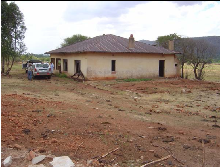
Fig.15 Farmhouse next to the S646 gravel road along the river. The building is unoccupied and is deteriorating rapidly at present.
