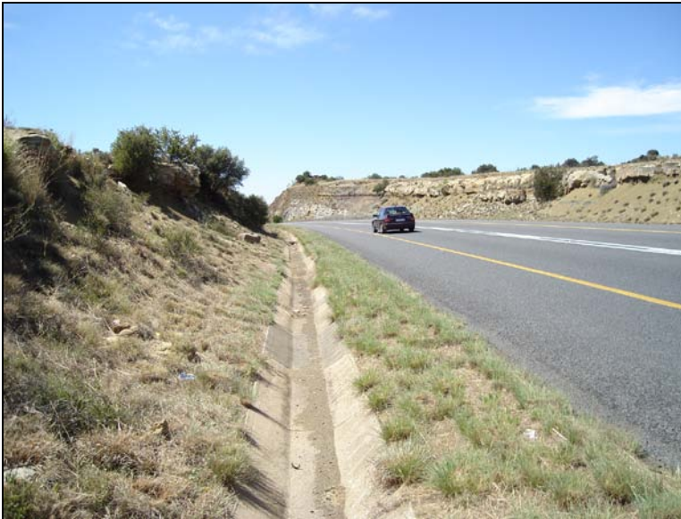
Fig.6 Road cutting at Km 36,3 on the N1 from Gariep Dam to Springfontein.
