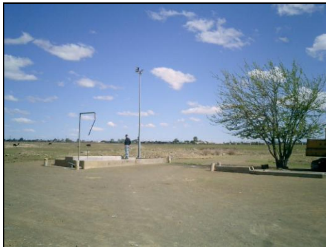
Figure 10: The existing inlet structure (IS), the upgrade of which will form part of the proposed development
