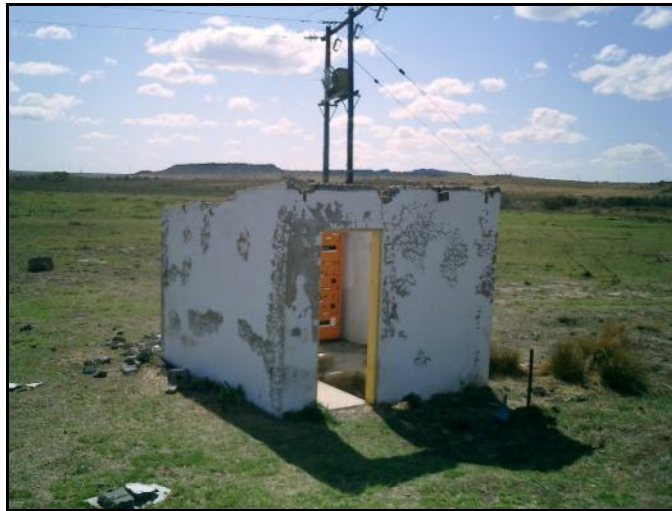
Figure 9: The R2 structure, post-dating 60 years of age and currently in use by the treatment works
