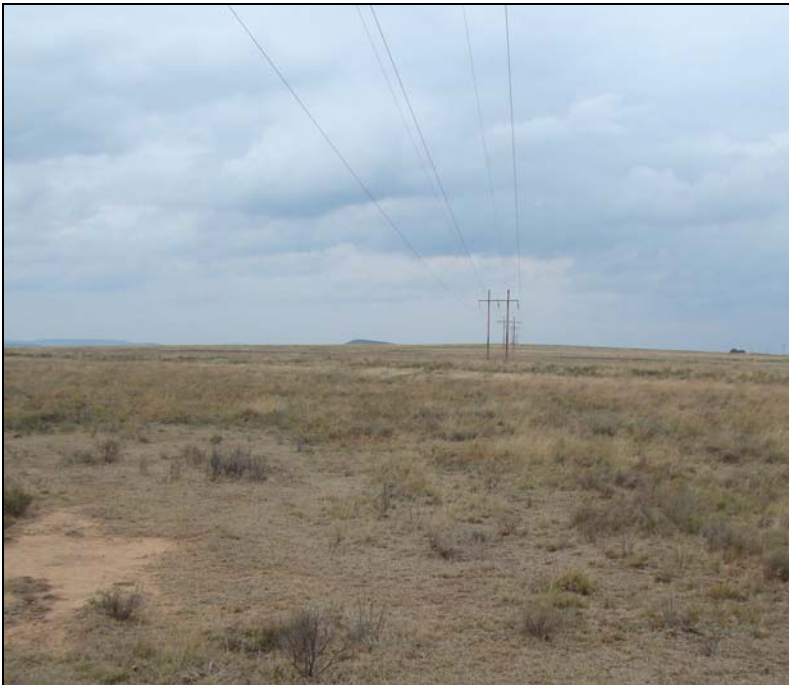
Fig.21 Pylon 19 on the Edenburg – Reddersburg line.
