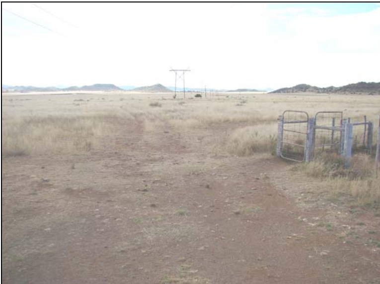
Fig.7 Pylon 128 on the Oranjekrag – Springfontein line.
