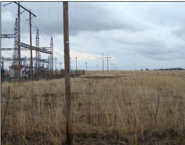
Fig.19 Pompie Sub-station on the Trompsburg – Reddersburg line.
