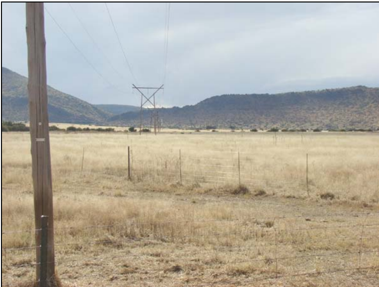
Fig.5 Pylon 55 at crossing with R701 road to Bethulie.
