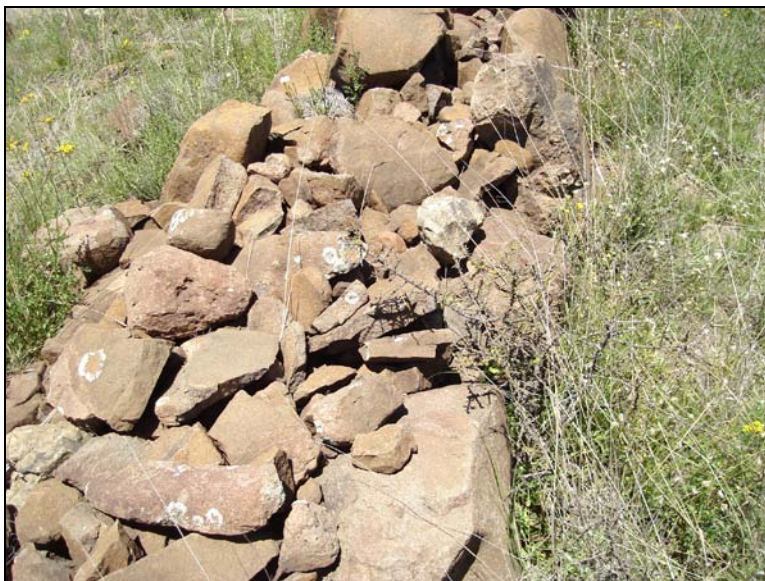
Fig.9 Detail of the construction of a stone-wall at Annex Elderslea "A" 433, Wepener.
