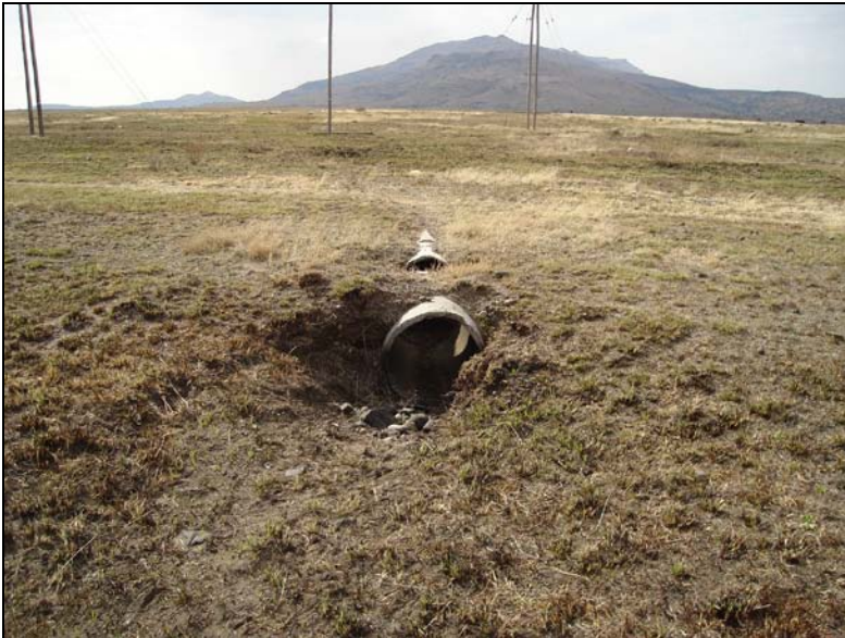
Fig.3 Remains of a culvert at the old road to Dewetsdorp that used to run through the area.
