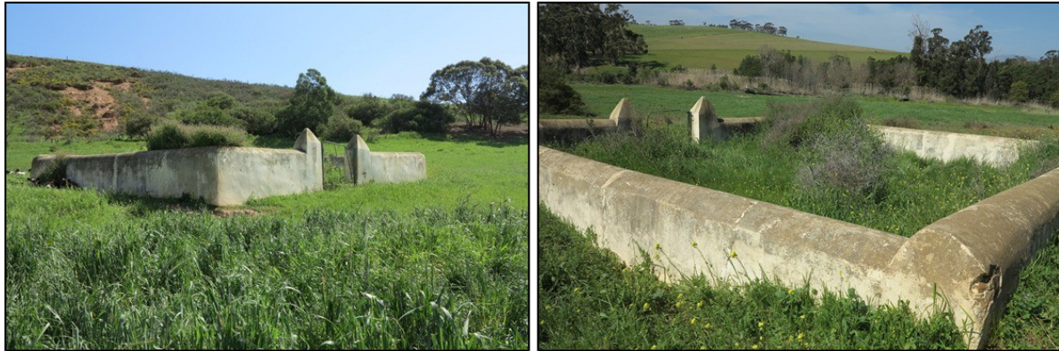
Figures 8 and 9: The overgrown cemetery - views towards the northwest and the southeast.
