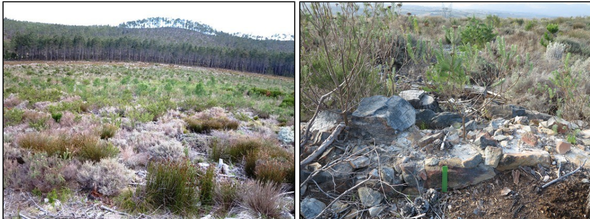
Figures 14 and 15: View towards the south showing the context of the foundation walls observed at the margins of the south-western corner of the proposed pit; detail of one of the best- preserved parts of the east-west running wall.
