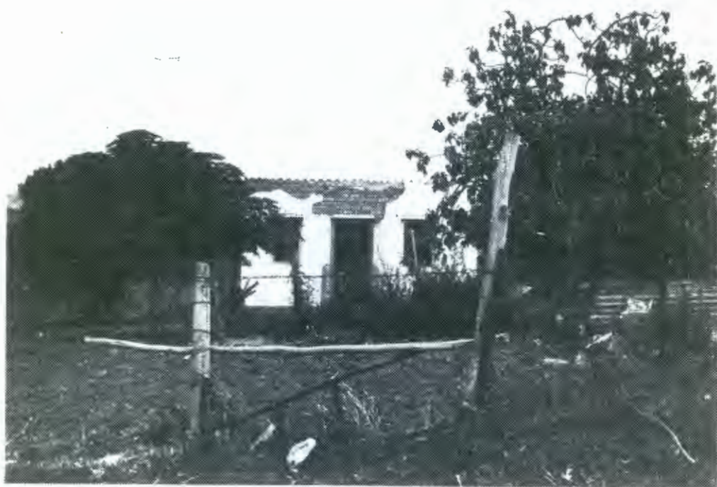
Semi-ruined cottage with corrugated iron monopitch roof. One 4-pane casement - door and other window missing.
