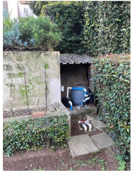
Figure P: Existing Pool Pump.
