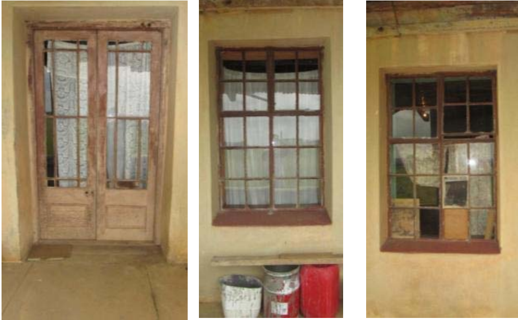
Figures 083to 085. External views of door and windows on the eastern veranda of house no 1. (P70, P71 and P72)
