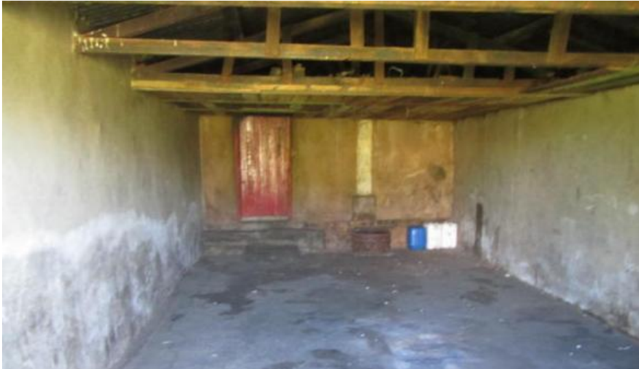
Figure240. Interior of garage showing signs of flooding and rising damp damage. Note the remaining veranda column and the unconventional carpentry in the trusses. (P131)
