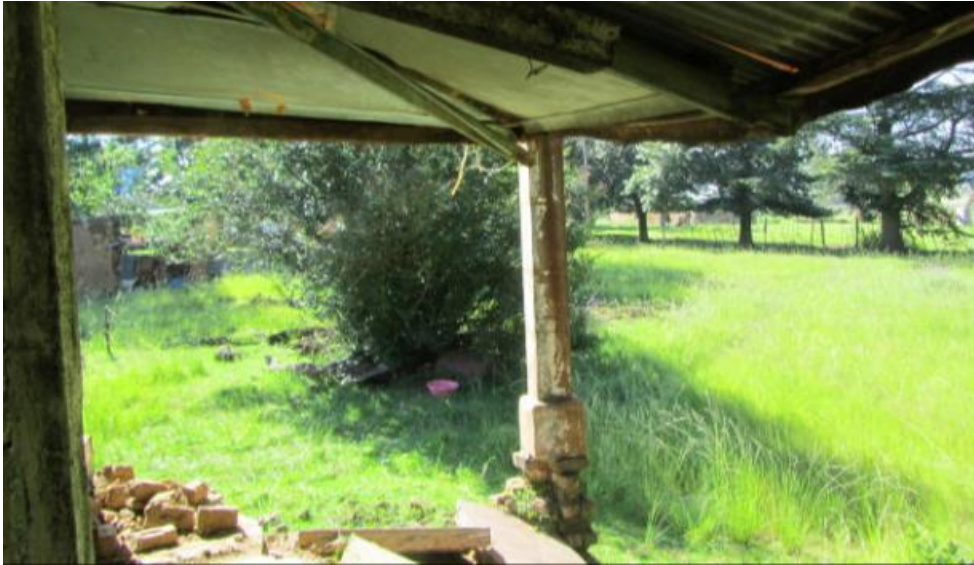
Figure 196. Detail of collapsed veranda. (P157)
