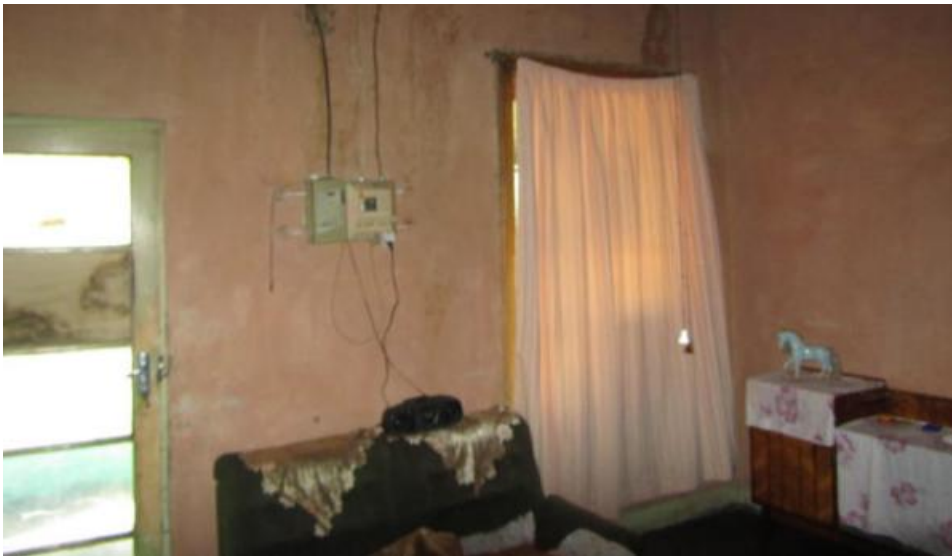
Figure 218. Electricity supply is modern and metered but rather dangerous. (P180)
