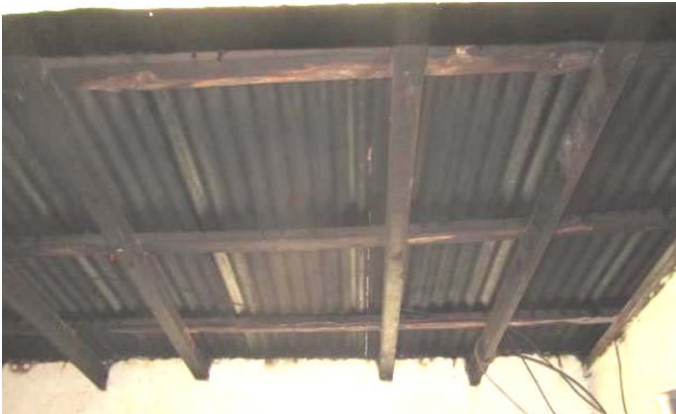
Figure 082. Northwards view of roof construction of the 'kitchen' of house no 1. (P69)
