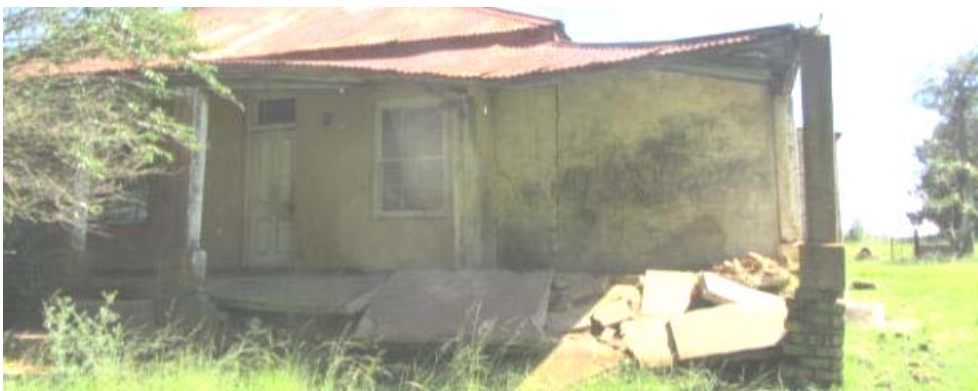
Figure 175. South elevation of the eastern part of the veranda showing conditions of imminent collapse. The reason for this is not clear as the veranda is not exposed to rainwater that may have contributed to the situation. (P121)
