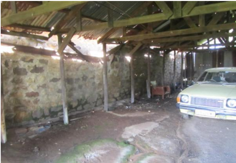
Figure 150. Interior of additional shed. Structure consist of modern 150 mm treated poles supporting individual trusses Note floor finish that consist of compacted soil and cement (Not concrete as illustrated by erosion caused by rainwater The purpose of this structure is unknown. (P42)
