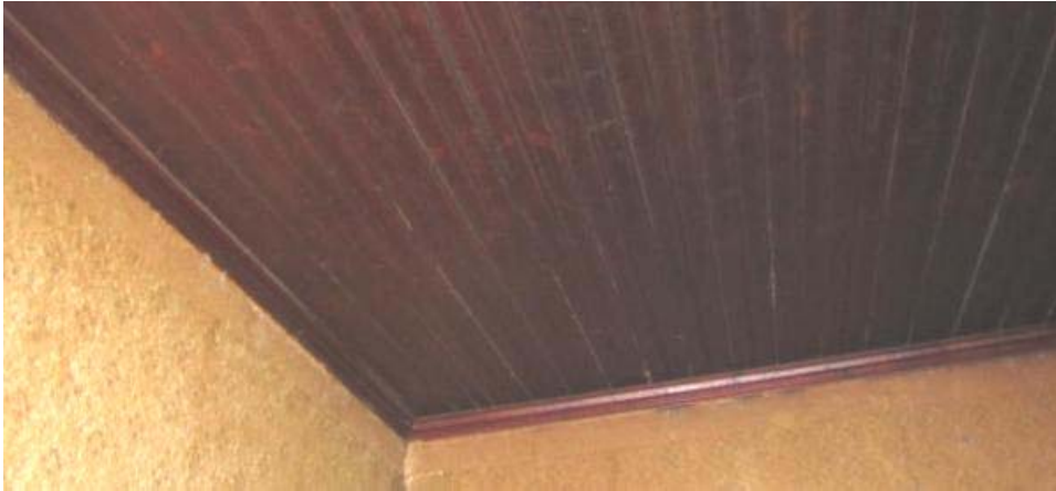
Figure 223. All internal ceilings were Edwardian double grooved pine. Some rooms shows signs of papering but most has been removed over time (P185)
