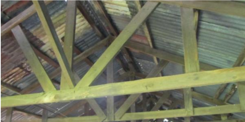
Figure 149. Interior of additional shed. Note modern pine used in trusses as well as unconventional carpentry. (P41)
