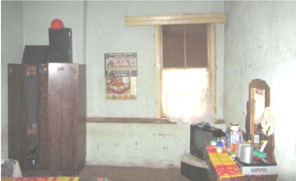
Figure 105. Note the difference in wall thickness adjacent to the window. This may be indicative of an alternative use before refurbishment. (P92)
