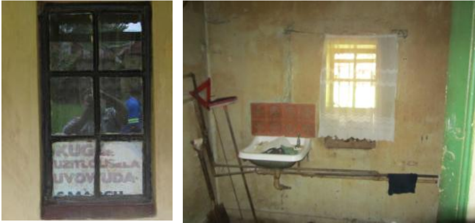
Figures 074 and 075. Two views of window in 'bathroom' in house no 1. (P60, P62)
