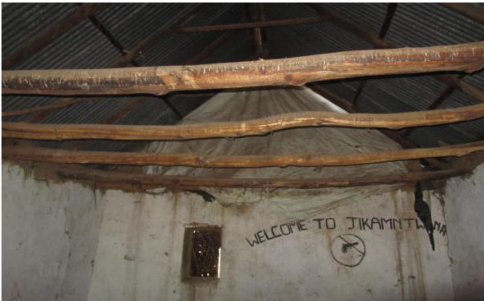
Figure 154. At present the wagon shed is used over week-ends as a community facility. Note the inefficiency of the trusses. (P46)
