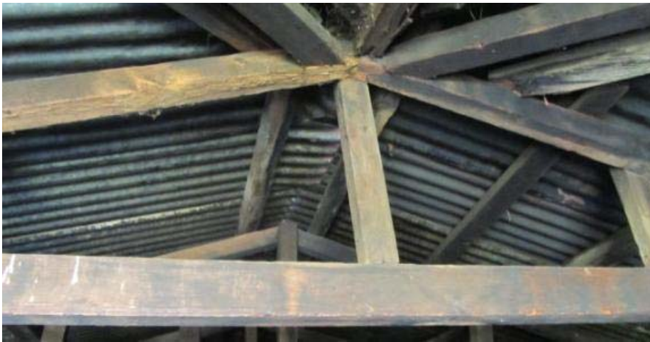
Figure 239. Truss detail of garage. The date of this addition is difficult to determine as it appears to consist of, 'modern' bricks and recycled wood and corrugated iron. (P130)
