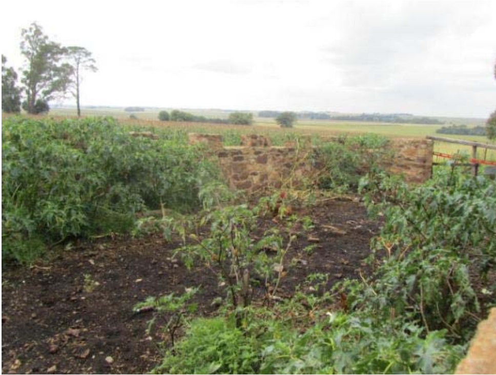
Figure 137. Dung build-up in the interior of the milking facility.(P31)
