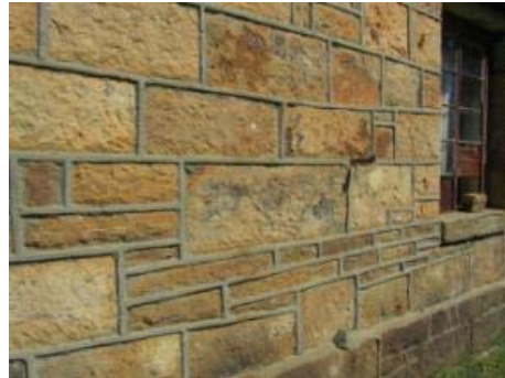
Figures 182and183. Looking eastwards from house no.2 and detail of pointed sandstone work.(P128 and P129)
