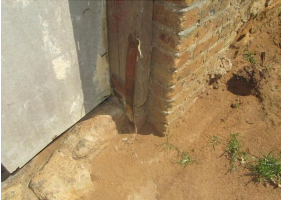
Figure 155. Detail of alteration to doorjamb and threshold. Bricks were utilized to repair stonework and to fix new frame. Threshold was built-up to avoid flooding of shed. (P47)
