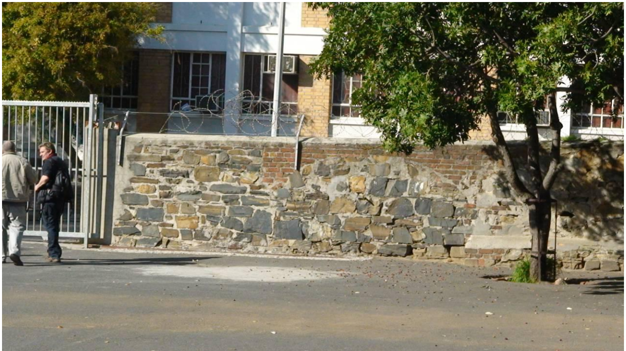
Figure 20. The old cemetery wall at Prestwich School. Parts of arched burial vaults have been included in school wall adjacent to erf 564 and Alfred Street.
