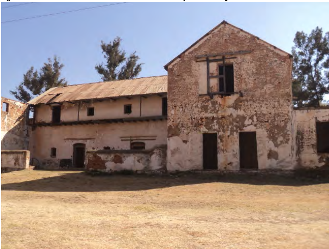
Figure 10. Cow shed with fire-damaged section on the left that housed the coaches.
