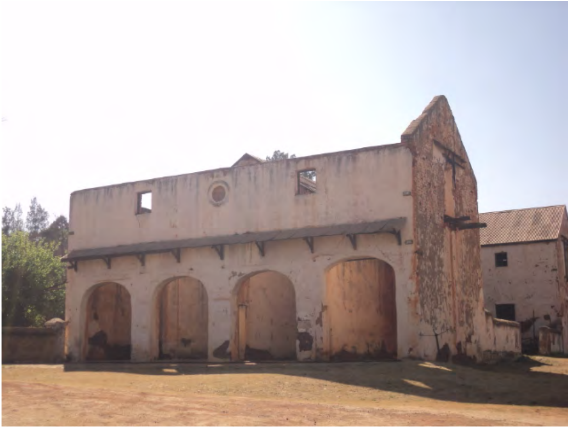
Figure 11. Coach building of which the roof was destroyed by a fire.
