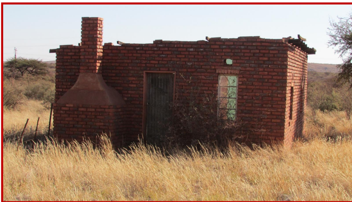
Figure 18: An overview of structure number four, this abandoned structure is also in poor condition, and has been looted on.
