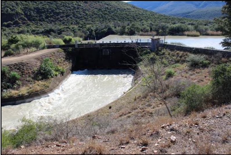
Plate 1: View of the Korhaansdrift dam and weir demarcating the beginning of the line route
