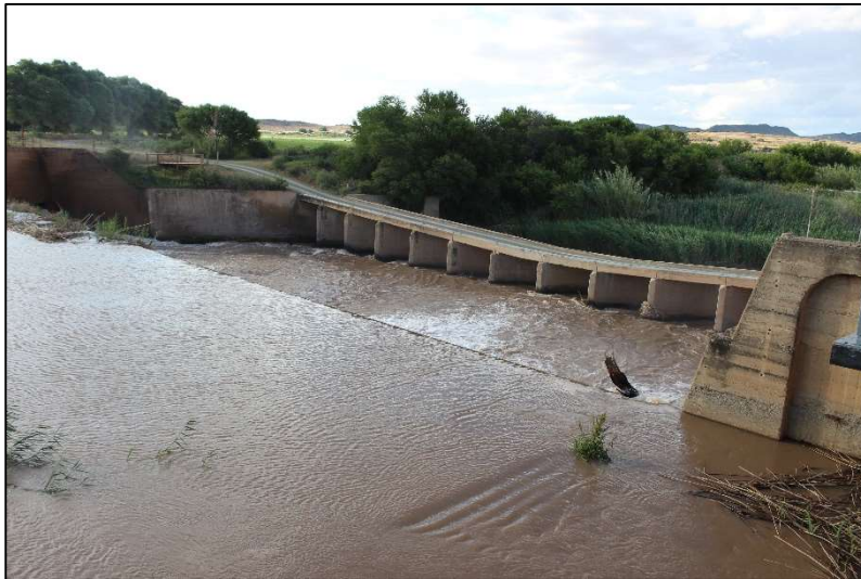
Plate 22: View of the bridge across the Great Fish River at the weir
