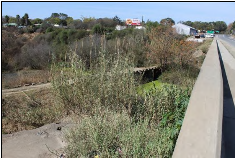
Plate 29: View of the Colonial Period Site FBA-S4 bridge from the B4301 across the Kat River [1]
