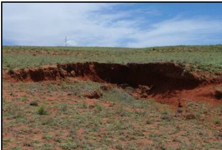
Figure 11: The TP3 erosion area with an exposed section of approximately 1.5m in height
