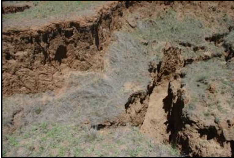
Figure 9: Erosion sections in excess of 5+m along the banks of the Tsomo River, south of the access road
