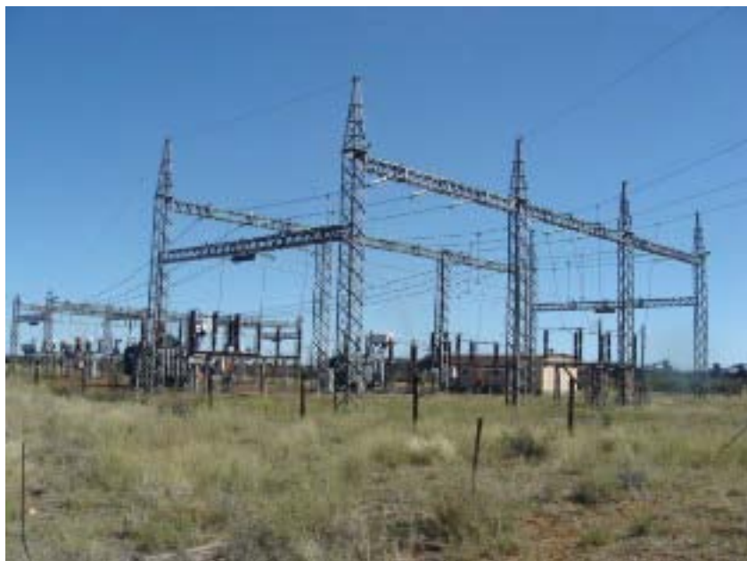
Figure 3: View of the ESKOM Substation in the area.
