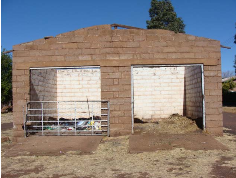
Figure 56 Garages also dating from a more recent period and currently being used for waste disposal.
